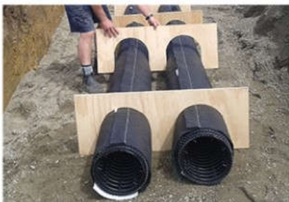
AES system pipes being installed in a sand bed by an AES certified installer.
